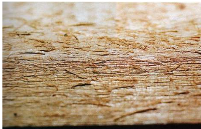
Figure 4. Fibres show the grain direction (here the grain direction is to the right)
